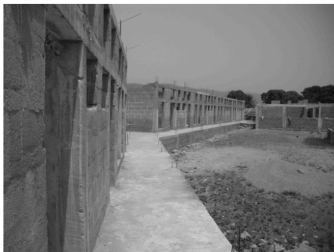
Figure 8. Current progress on construction of new Lassa Ward. This is the view from the rear of the High Containment wing, with the Administration Building on the right. Construction is projected to be complete by August 2014 (photo credit RFG; 28 Feb 2014).
